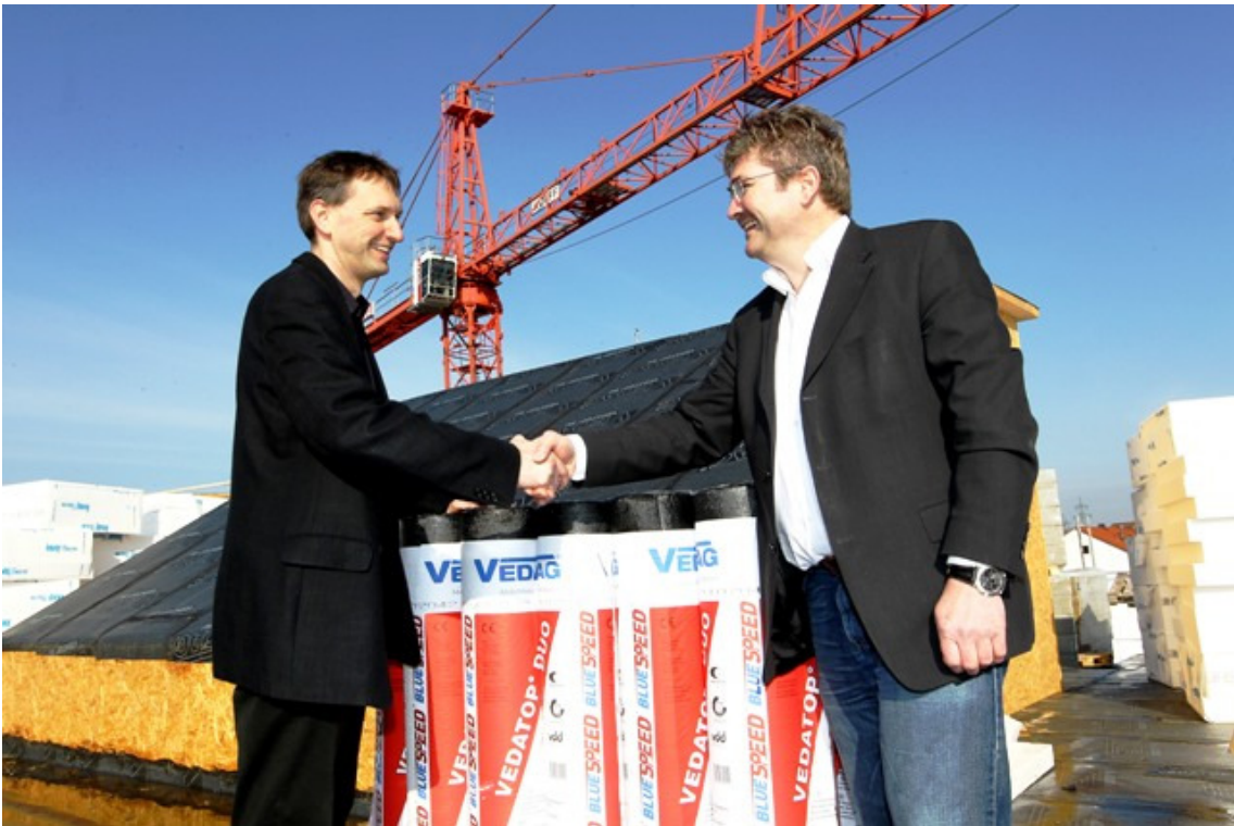
Johannes Kalusche from VEDAG GmbH (right) and Ralf Göller, head of building services /construction subproject head from Stadtwerke Bamberg, confirm the good collaboration on-site. Source: Stadtwerke Bamberg
